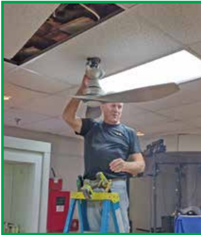
The First Marine Detachment helped out. Here is Bob Broderick installing ceiling fan in game room.
