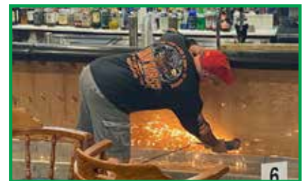
Jeff Cwynski removing the facing of the bar so it could be replaced with an upgrade.
