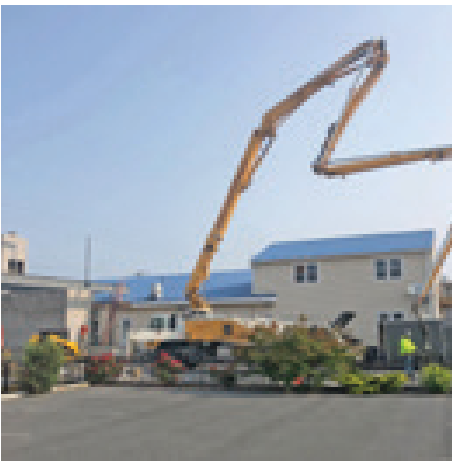
That's not a new Trimper ride. It's how the construction crew got the concrete to where it was needed
